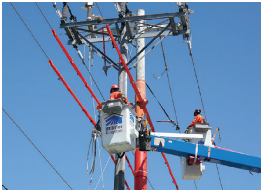
Customers of Utilities Kingston benefit in multiple ways from its innovative multi-utility model. Photo courtesy of © Paul Wash.
